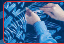
Structured Cabling & Telecom Solutions
